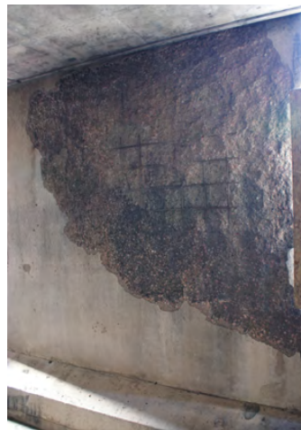
Spalling observed after a fire in a parking garage. Courtesy of Robert McNamee.
