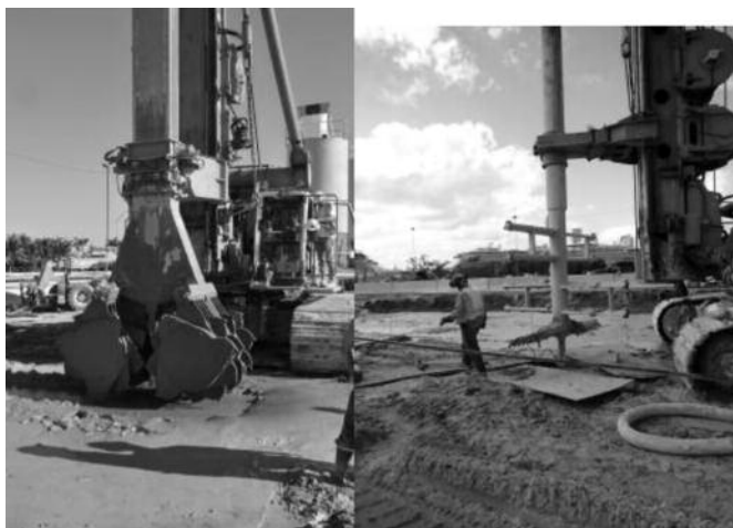
Fig. 3. CSM Cutter & Renforcement de sol de surface (SSM) / CSM Cutter & Shallow Soil Mixing (SSM)
